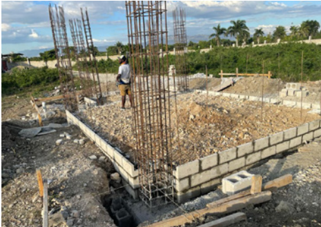
Starting work on the Generator/Water Building. Note the cap of the water well in the upper left of the photo.
