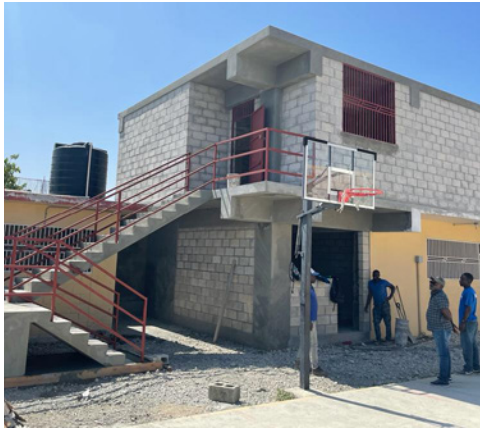
Completion of the 2nd floor, Youth Building, Repatriote. Painting and interior finishes are still needed.
