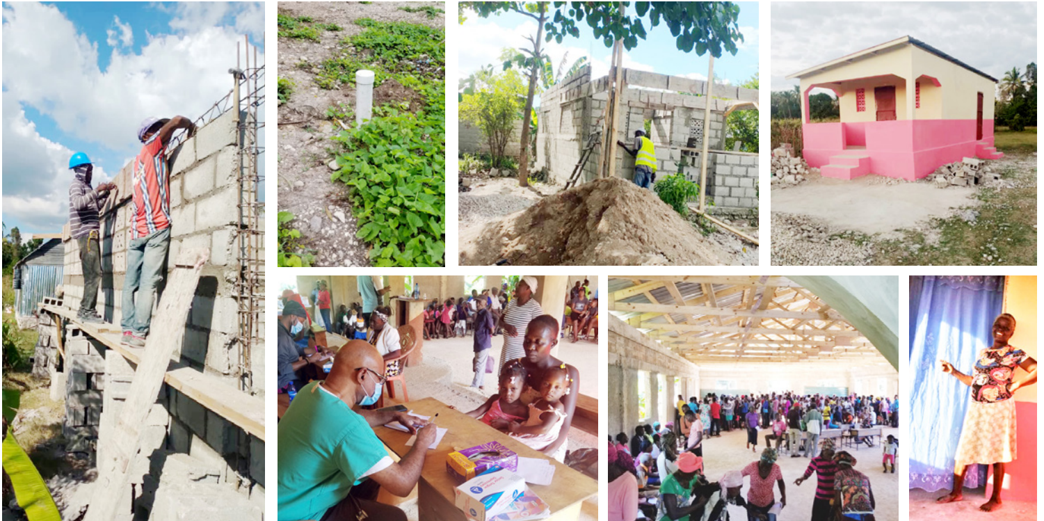
Top row: Home construction in progress, early stages of a new well, and a completed house. Bottom row: A busy mobile health clinic in action, and a happy new home recipient.
